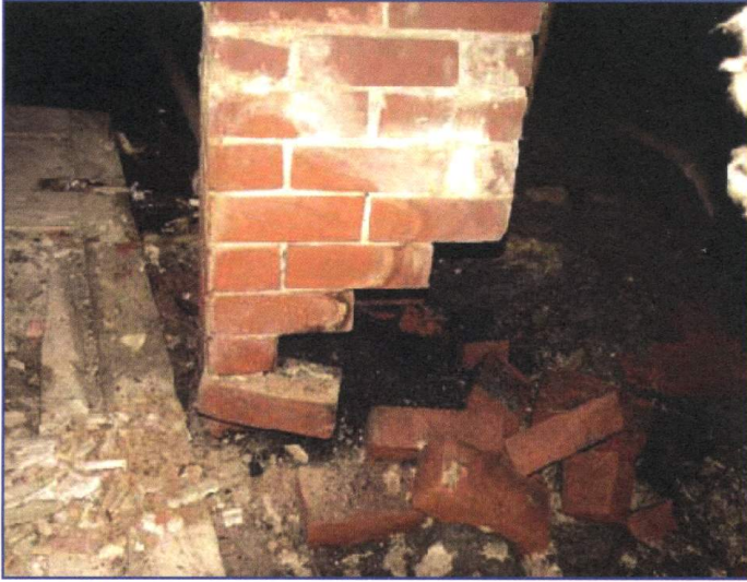
Air will take the path of least resistance in or out of the chimney based on pressure differences.
