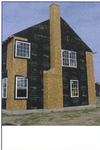
CHIMNEY CHASE: An insulated chimney chase reduces heat loss from a chimney. The insulation should be installed when it is built.
